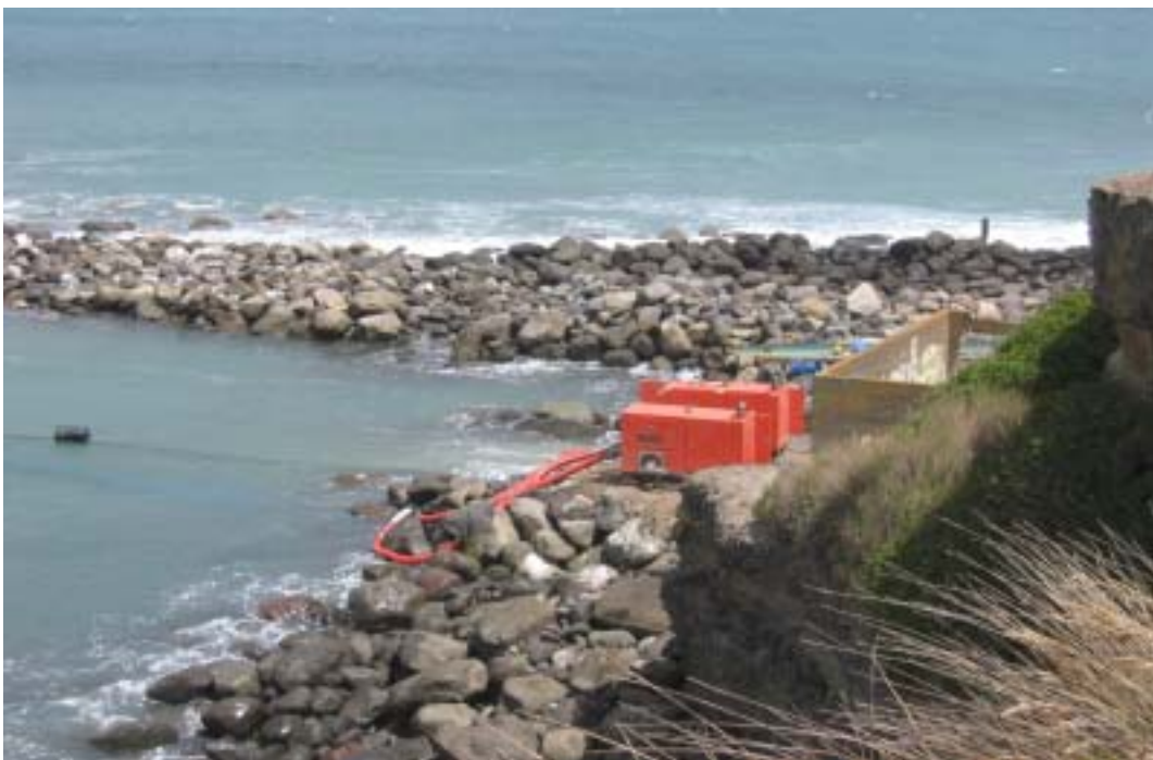
Photograph 5 Sand pumping equipment
