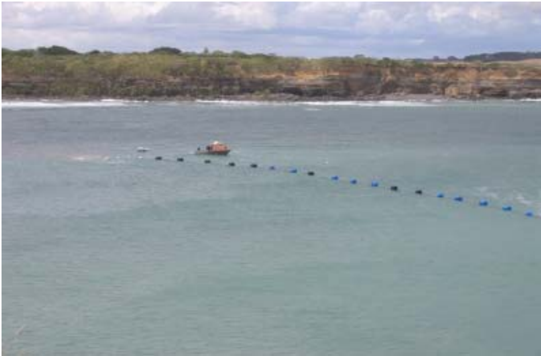
Photograph 4 Buoys float the pipe used for pumping the sand slurry mix out to the geo-textile bags
